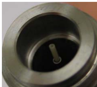
Sample line installed incorrectly
